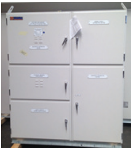
Figure 1: DaRa main switchboard for Baptcare aged care redevelopment project
