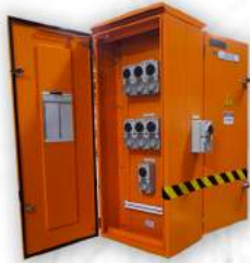
Temporary Power Boards
