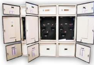
Group Meter Panels
