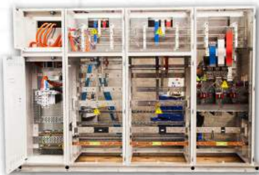
switchboards for PV power plants
