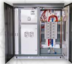
Automatic changeover switchboards
